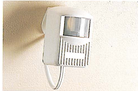
Passive Infra Red alarm system
