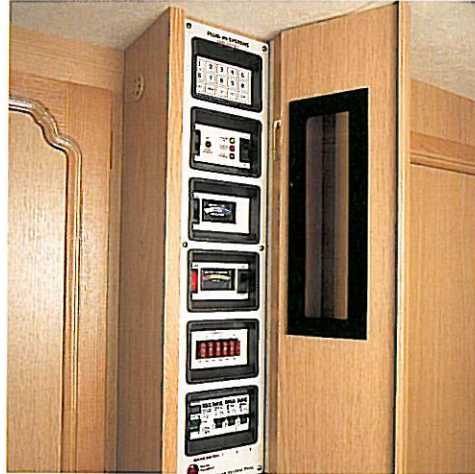
Modular electric control console
