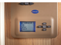
Alde central heating system
